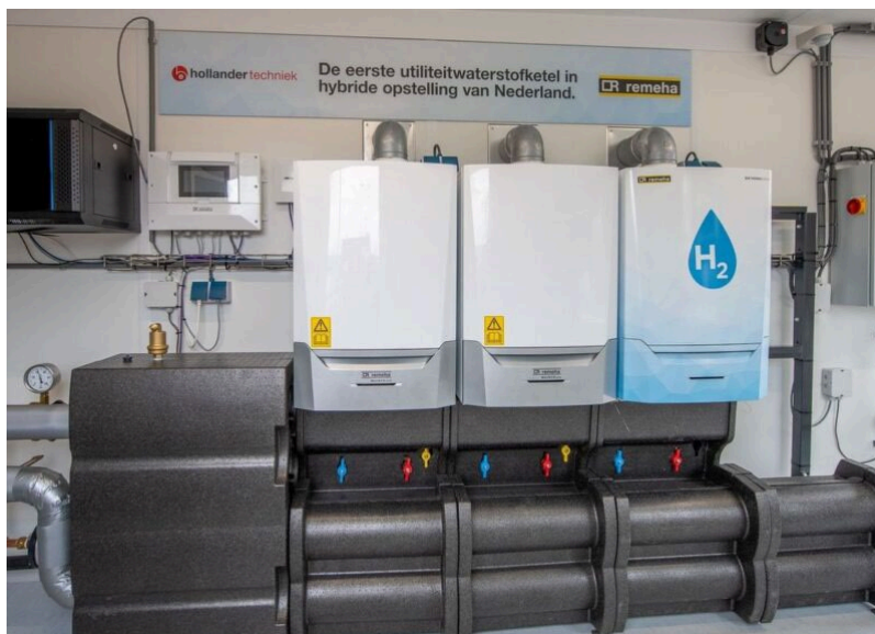
Figure 5. Hydrogen heating boiler integrated into the heating system of an office building [22]
