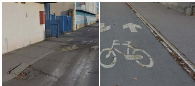
Figure 15. Damage and demarcation of the pedestrian and bicycle path
